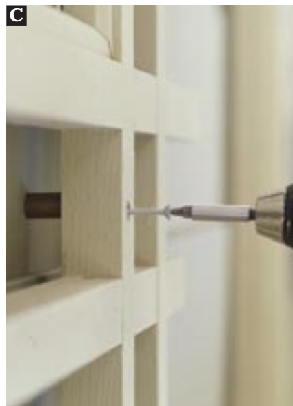
Attach all four mounting screws loosely at first, then snug them down to hold the trellis firmly to the wall.
